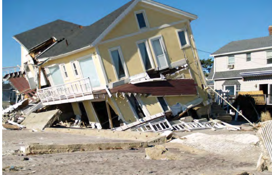
The dramatic impacts from Hurricane Sandy in 2012 illuminated the need to more closely coordinate the management of sand resources across jurisdictions in our region. A property in the Rockaways, New York that was damaged as a result of that storm captures the sense of urgency. © NY DEPARTMENT OF STATE
