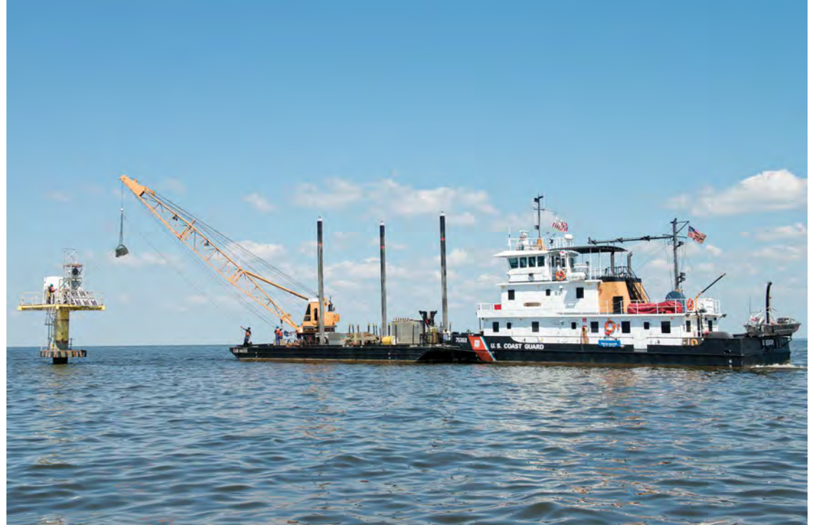
Crewmembers aboard Coast Guard cutter Sledge use the ship's crane to lower a new transformer down to Craighill Entrance front range light Aug. 25, 2014. Crew members from Aids to Navigation Team Baltimore help guide the transformer onto the structure by use of the tag line.
