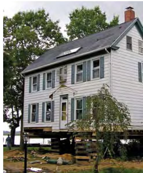
Storm damaged house being raised above base flood elevation. (Photo: Harriet and Bud Hankins)
